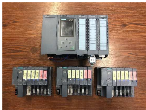
Figure 4 : PLC system for the gas control, with the CPU, I/O cards and ET200SP remote I/Os
