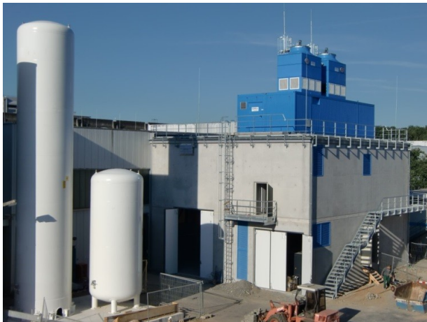
Helium tanks and annex building with 1,1 MW water cooling
