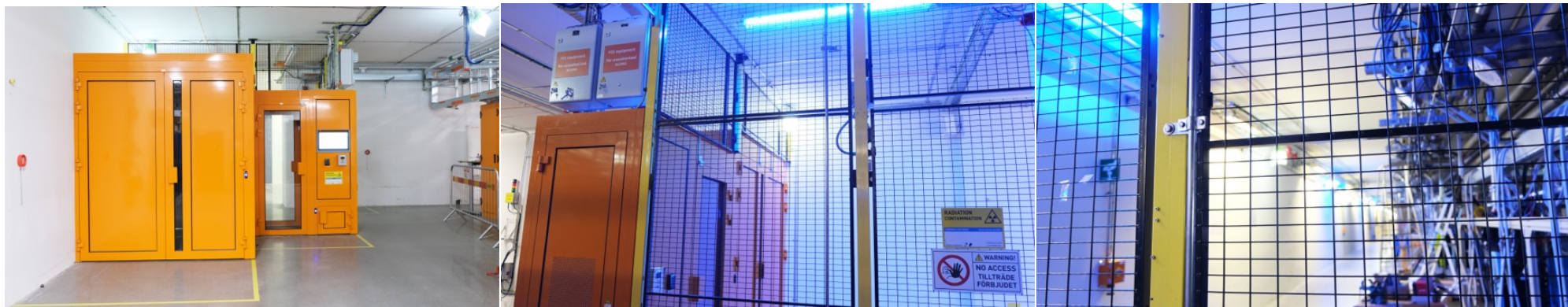
Personnel Safety Systems installed in Front End Building.
