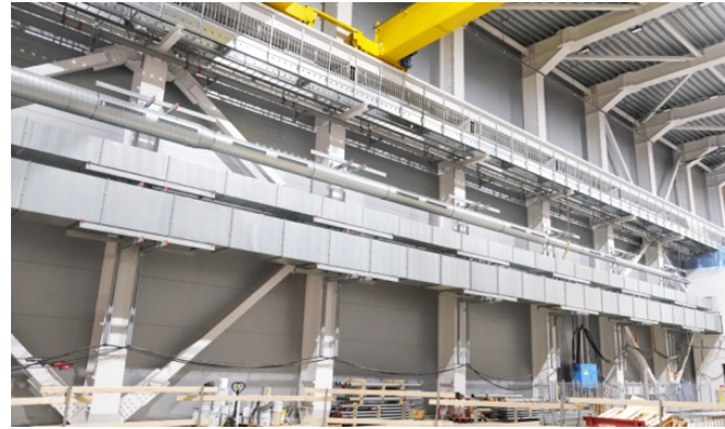
High bay: Ventilation ducting and piping.
