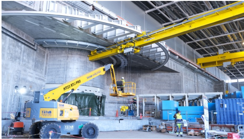
D03 overhead crane commissioned, and bunker crane installed
