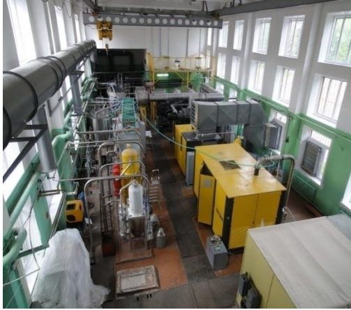
Hall of the cryogenic equipment
