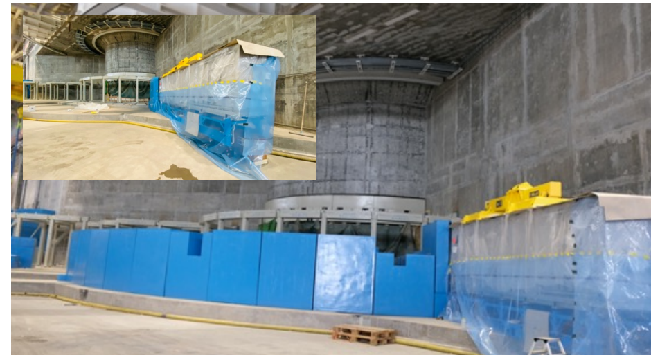
Estia Selene 1 Guide housing delivered to D01
