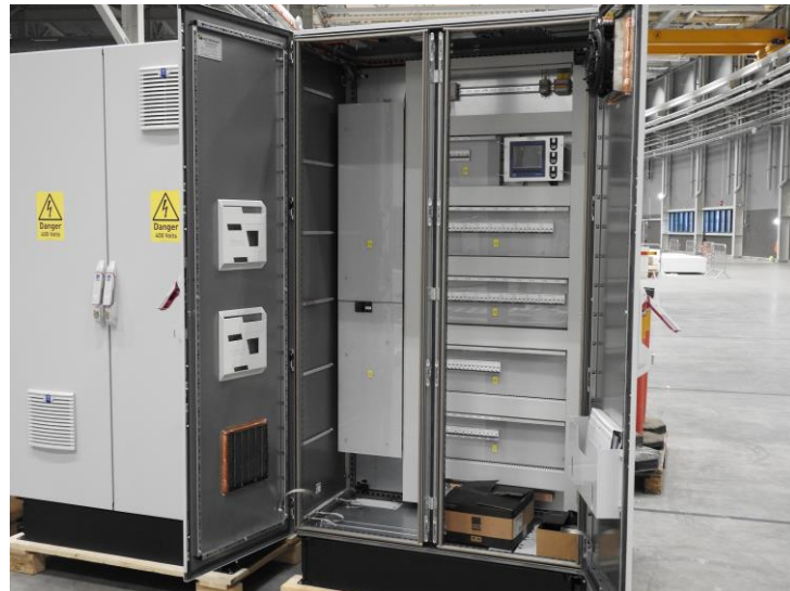
MIRACLES Distribution Board
