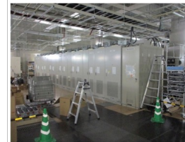
QDN power supply into D2 (Chopper + Filter + Control Panels)
