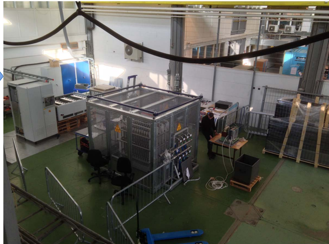
Larger test stand (130m 2 ), for high power testing (160 kVA)
