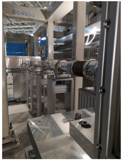
ODIN in-bunker installations
