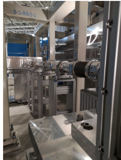
ODIN in-bunker installations
