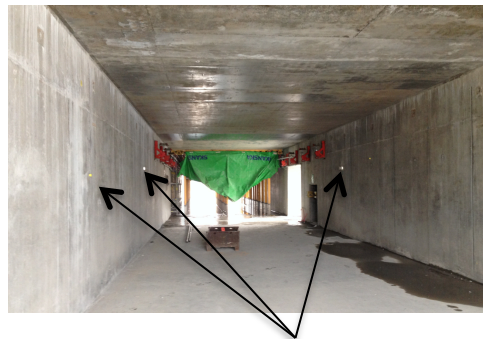
Tunnel network references already installed.
