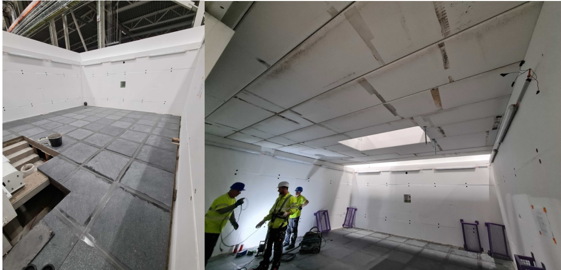
Figure 1: (left) granite tiles installed and ready for polishing. (right) experimental cave roof installed, and fences delivered.
