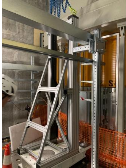
Figure 1: Pulse shaping chopper remote handling frame installed inside the bunker.
