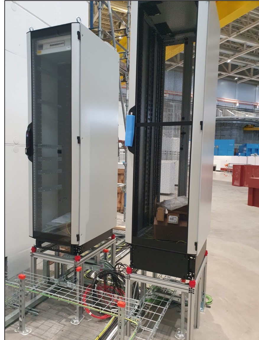
Cabinet frames install at DREAM
