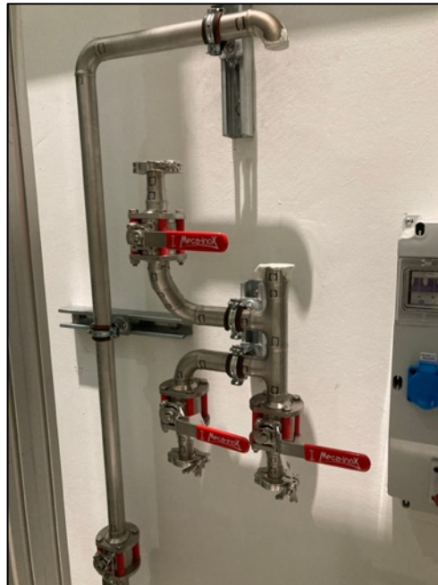
Utility panel inside the cave
