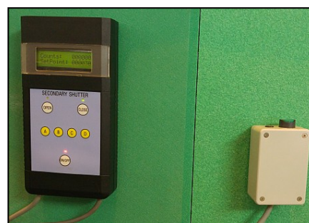
Figure 9. Interlock box and emergency exit button.
