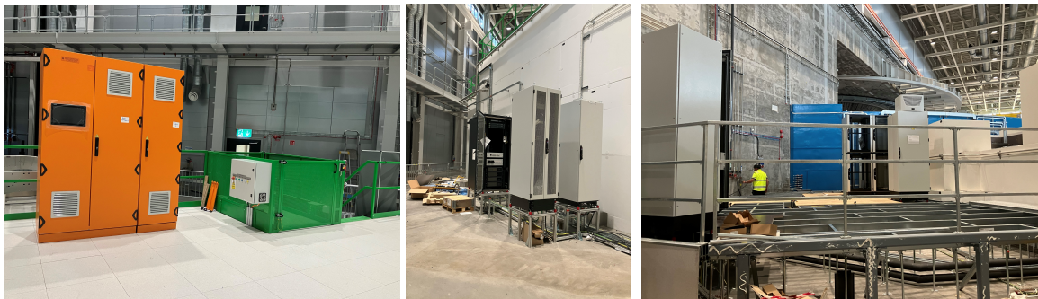
Figures 1: PSS cabinets on DREAM elevated floor – ICS, Vacuum and Master & Slave Detector racks behind the cave. The surrounding elevated floor is scheduled for November. – The chopper racks in the South bunker area.
