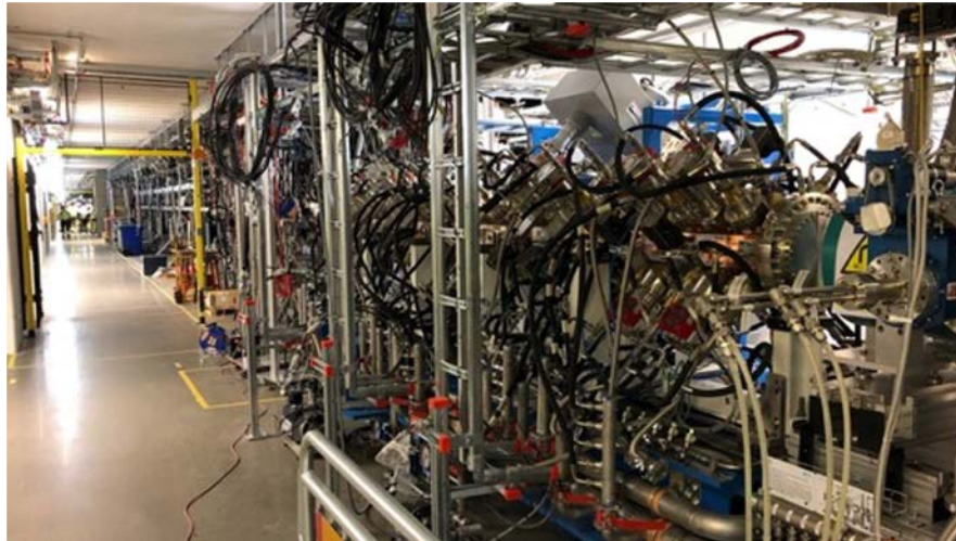
Parts of Normal Conducting Linac Under commissioning
