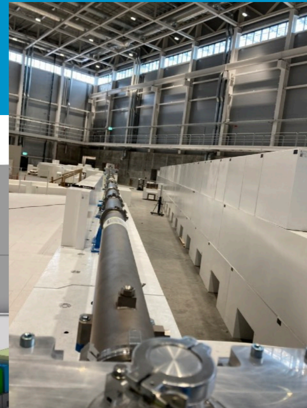
In-kind from Hungary, installed Feb 2024
