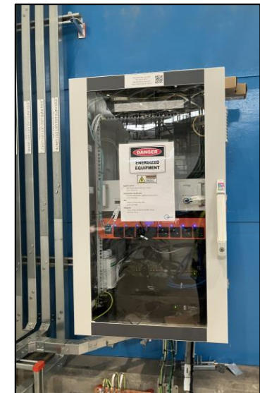
Rack for M1 system electronics
