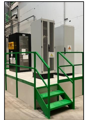
Rack for M3 system electronics (Detector rack)
