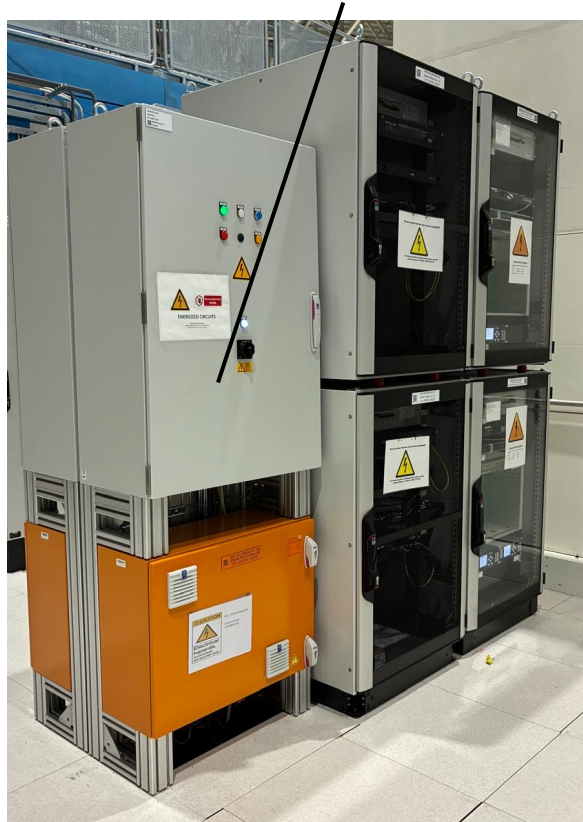
Shutter control rack in bunker rack area
