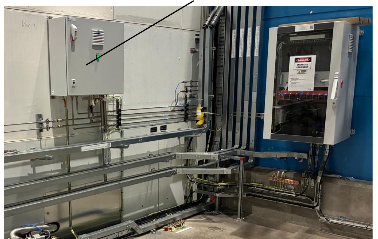
Shutter pneumatic rack close to bunker
