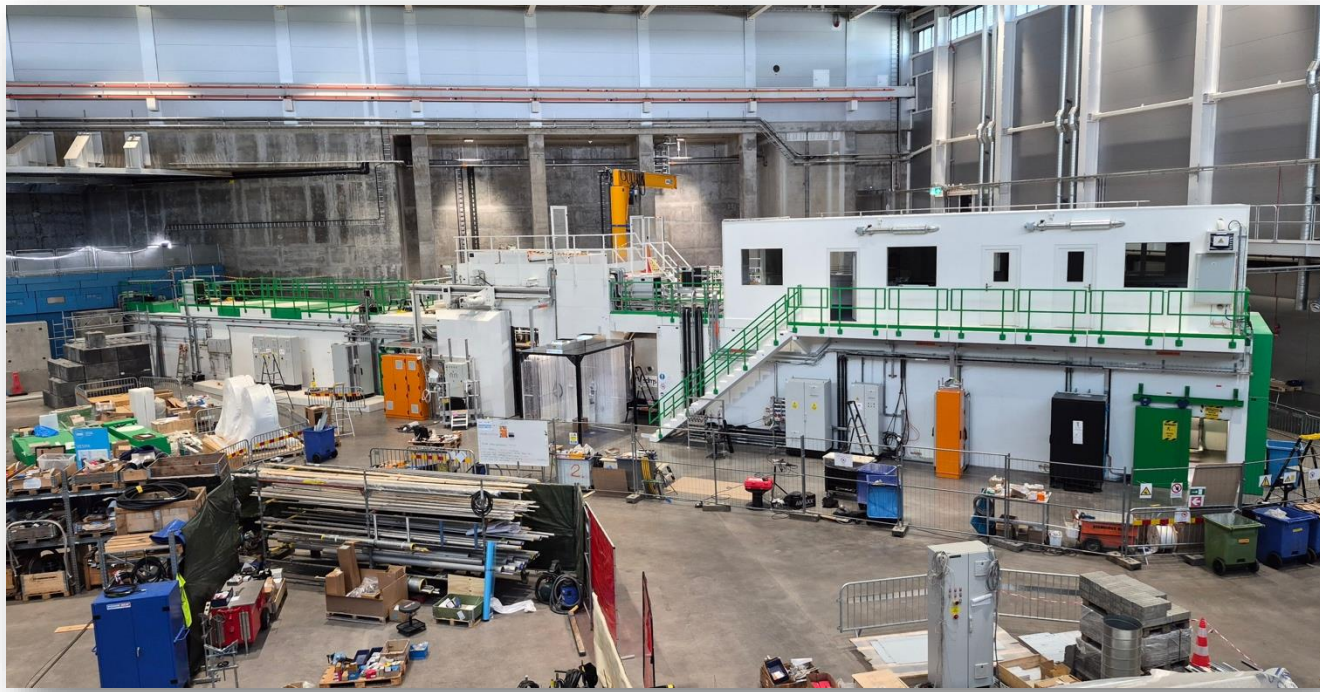
Cave, Collimator Shielding, and Hutch Installed Electrical and Utility installation started. Detector vessel delivered and installed
