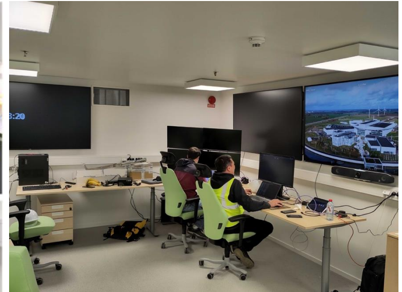
Control Hutch fitted out and in use for training and testing
