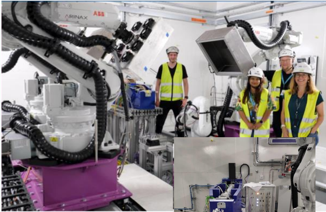
Sample and detector robots installed and undergoing inspection for energisation
