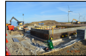
Photo 1, Cable Pits G04
