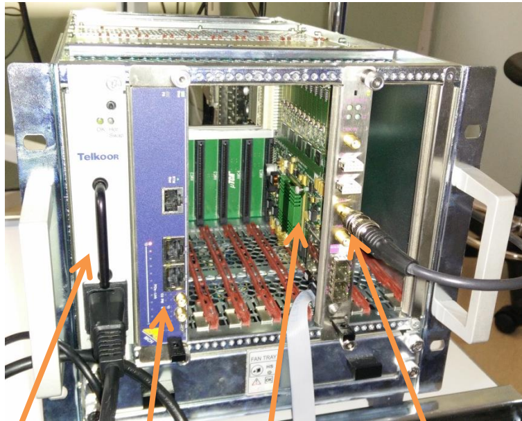
Power supply unit microTCA.4 MCH Struck SIS8300-L2 board Input clock signals
