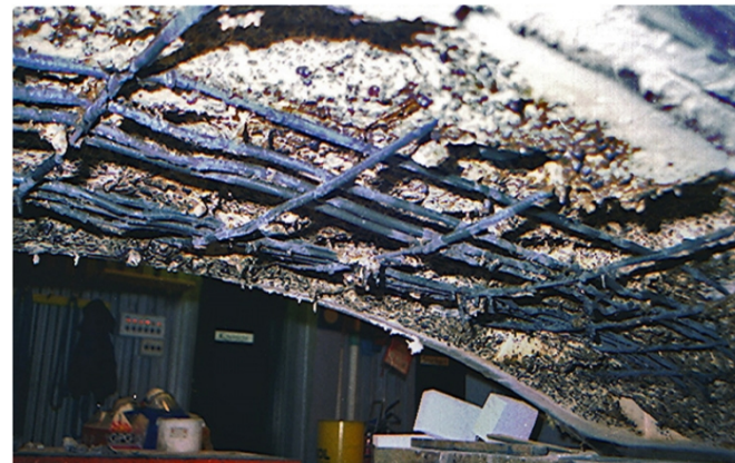
Tunnel element from the Great Bealt tunnel fire tested at SP Technical Research Institute of Sweden.
