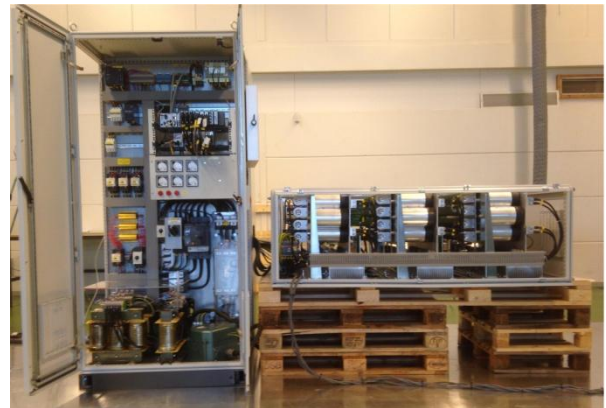
Figure 6: View of low voltage converter stage cabinets.
