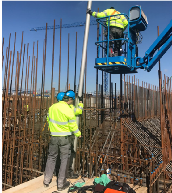
Figure 4: High electrical conduits installed for embedment into Active Cells floors and walls.
