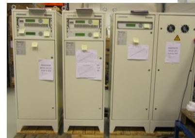
Large 4 cabinet power supply
