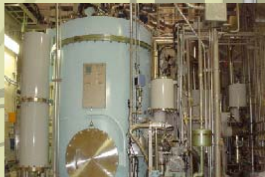
Cryogenic hydrogen system
